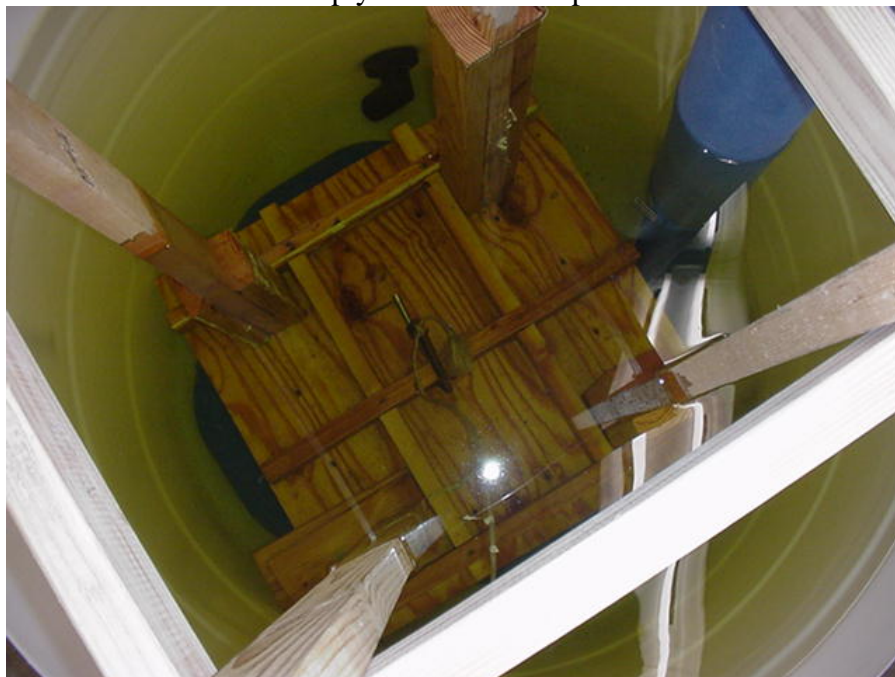
Under water view of reinforced plywood shored in place to restrain the test mockup
