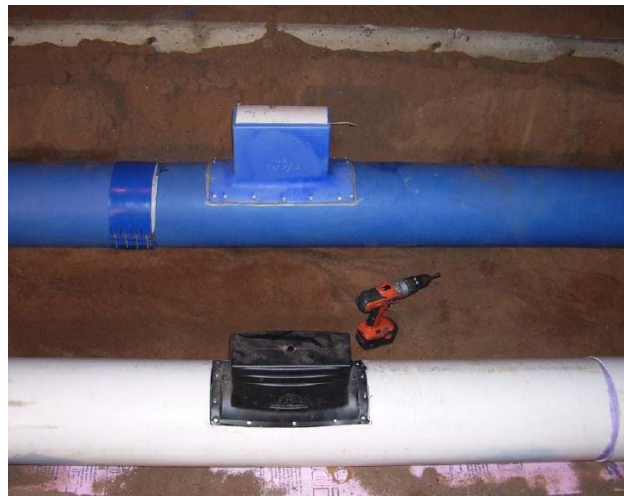
Register attachment to the two duct systems
