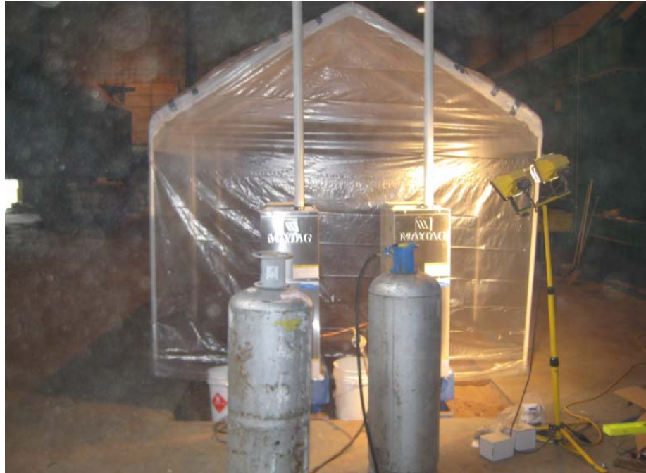
The identical furnaces outside the test room each with 100 lb LP tanks
